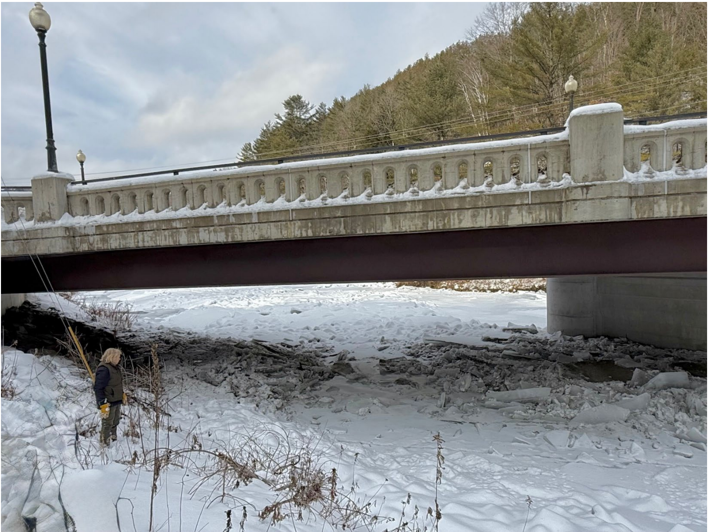
Photo 1 Tunbridge Volunteer Fire Department Drafting Site is blocked by an ice jam.
